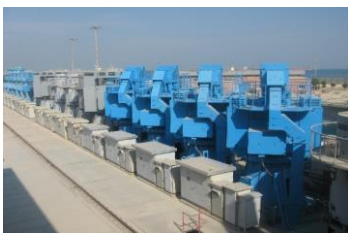
Figure 1. Part of the pumping station under study
