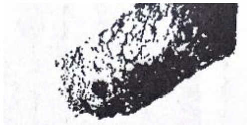
Figure. (1-A) : Concrete slab corrosion from not using trapped air additives
